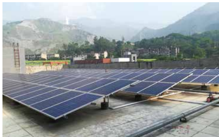
Rui'neng Solar Power Rooftop Project in Sichuan, China
