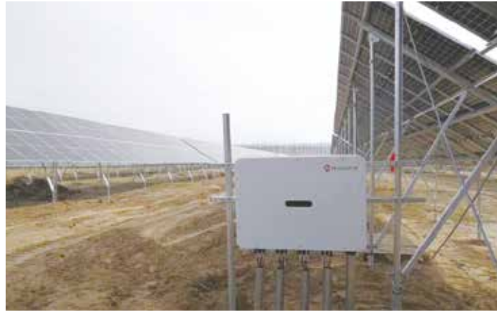
200MW hopeSunHV250KTL Utility Project in Ningxia, China
