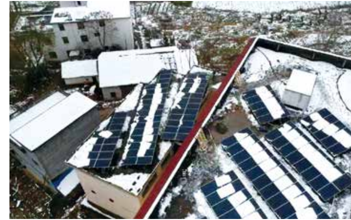
Solar Power Project in Jiangxi, China
