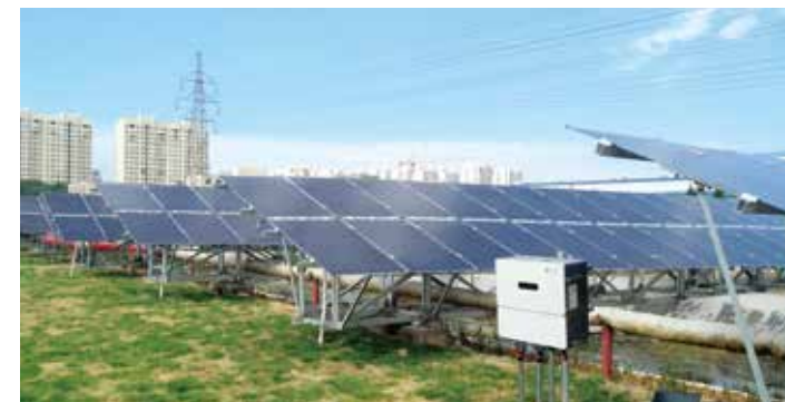
CNNC 2.8MW PV Project in Shandong, China
