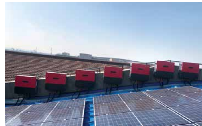
Rooftop PV Project in Jiangsu, China
