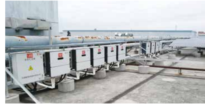
Roof-top Project in Jiangsu, China
