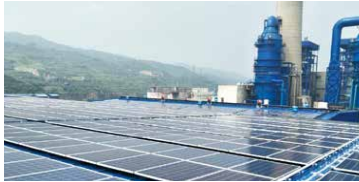
Operation of 50kW String Inverter
