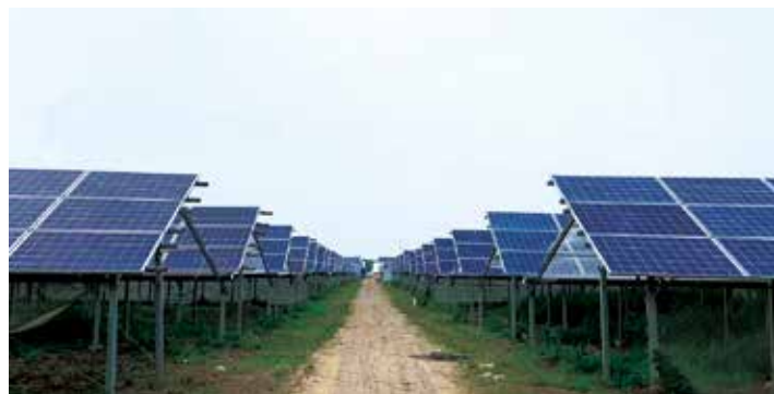
Solar Renewable Project in Anqiu, China
