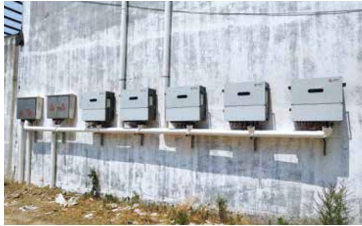
Rooftop PV Project in Shandong, China
