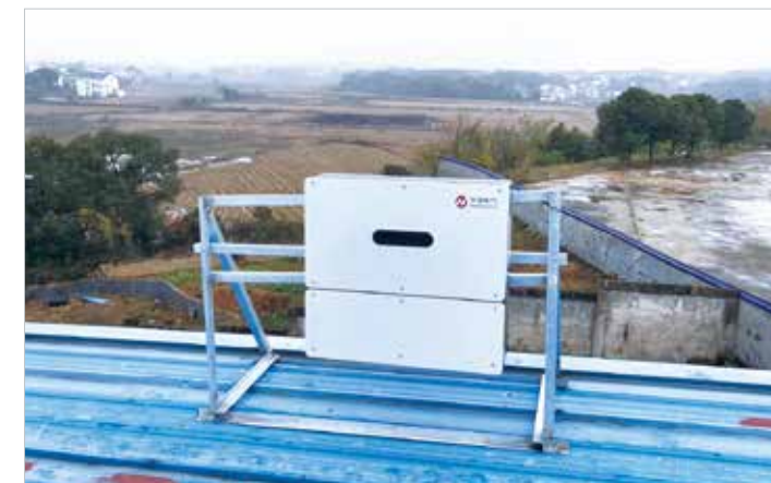
Rooftop PV Project in Hunan, China
