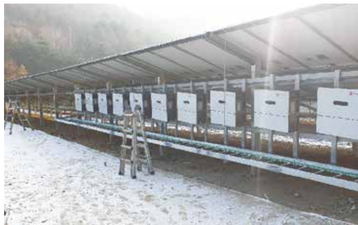
550kW Solar Plant in South Korea
